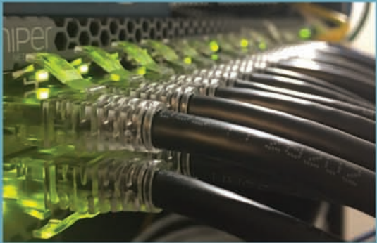
Structured Cabling Solutions
