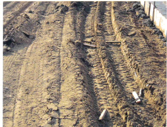
Example of failed subgrade
