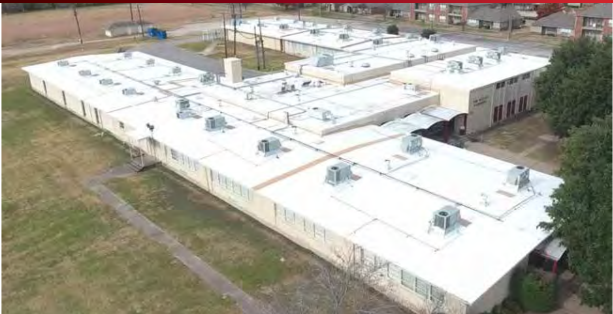
Ennis ISD - High School - Installed in 2019
