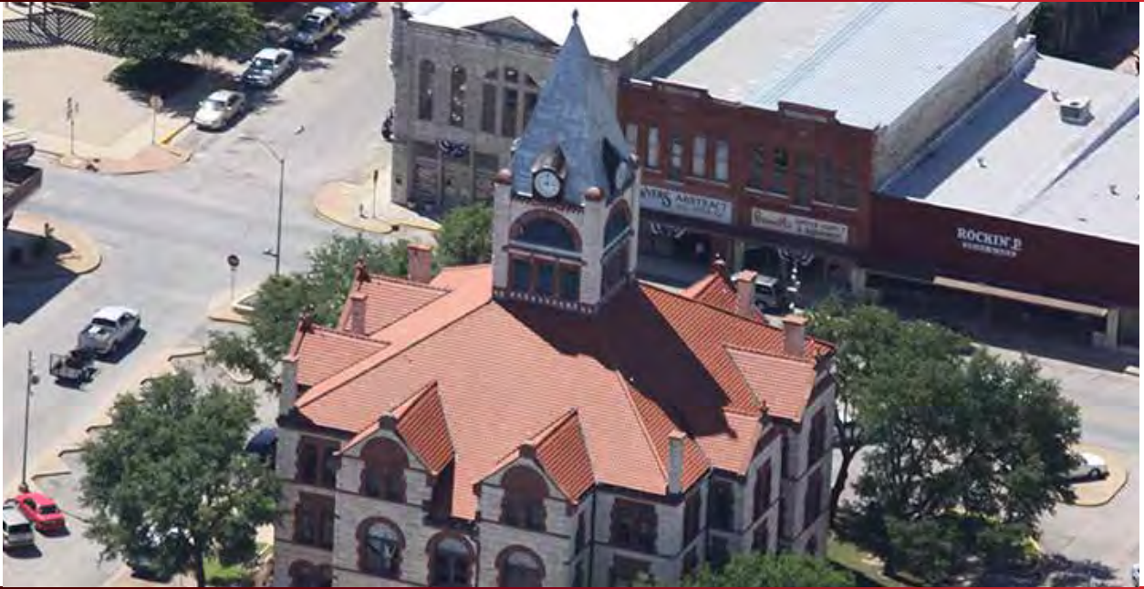
Gillespie County Courthouse - Installed in 2009
