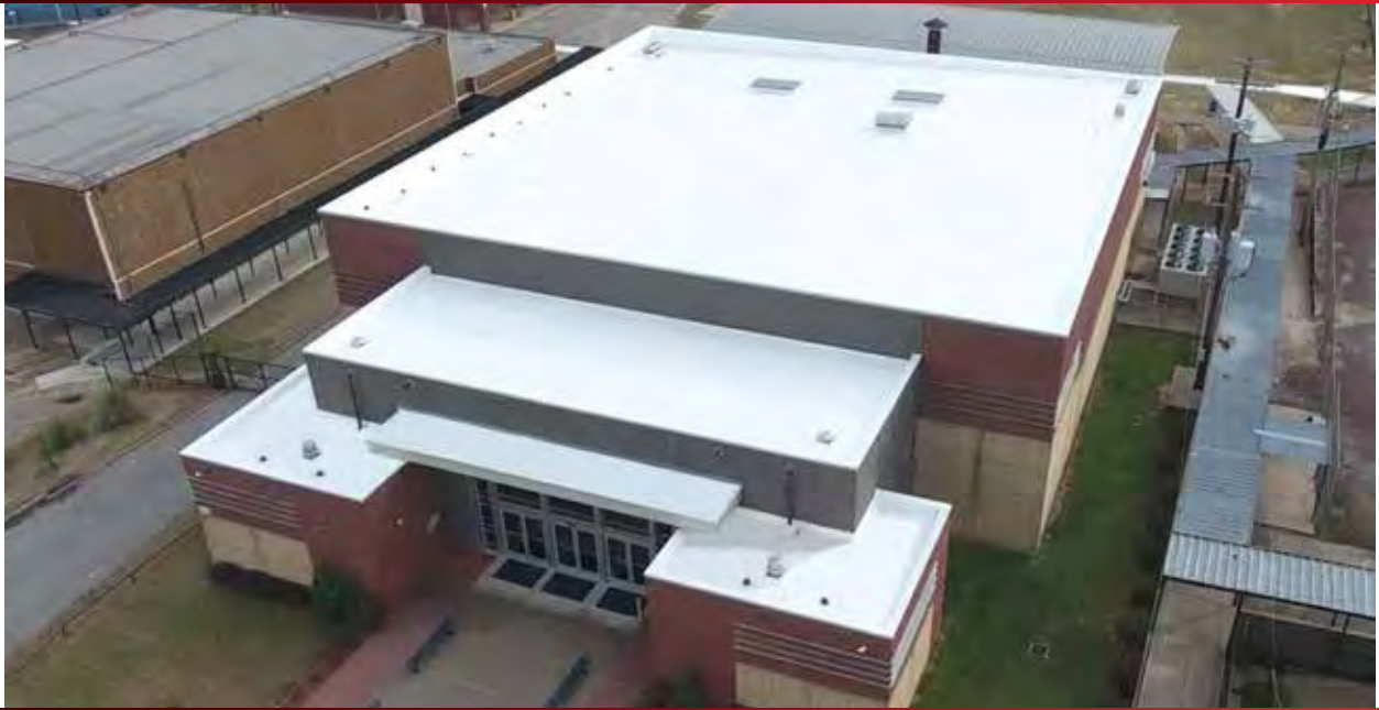
Overton ISD - Installed in 2010
