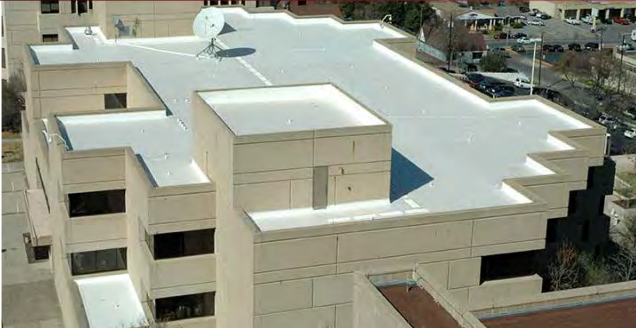
University of Texas - Arlington, TX - Installed in 2011
