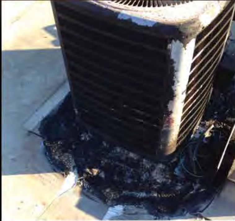
Duro-Last System at Fort Hood saves roof from AC unit fire.
