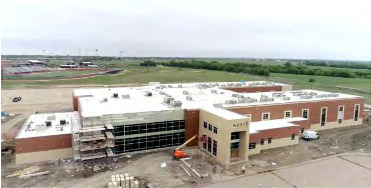
Midway ISD - Chapel Park Elementary - Installed in 2022
