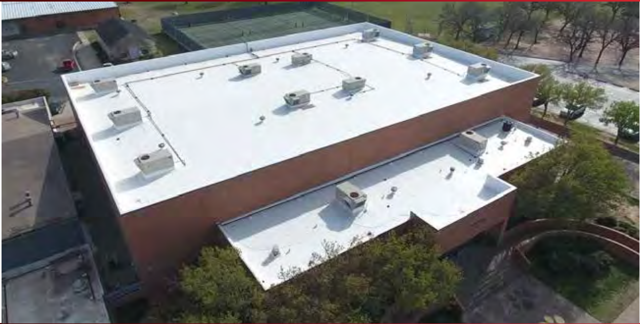
Clyde ISD - Junior High - Installed in 2010
