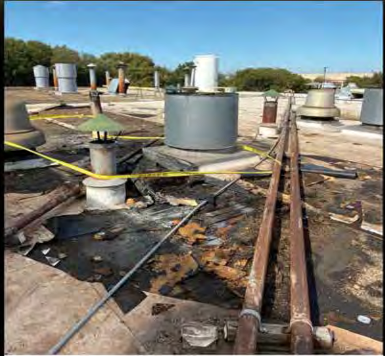
TPO System at Texas Heat Treating burns and continues to spread.
