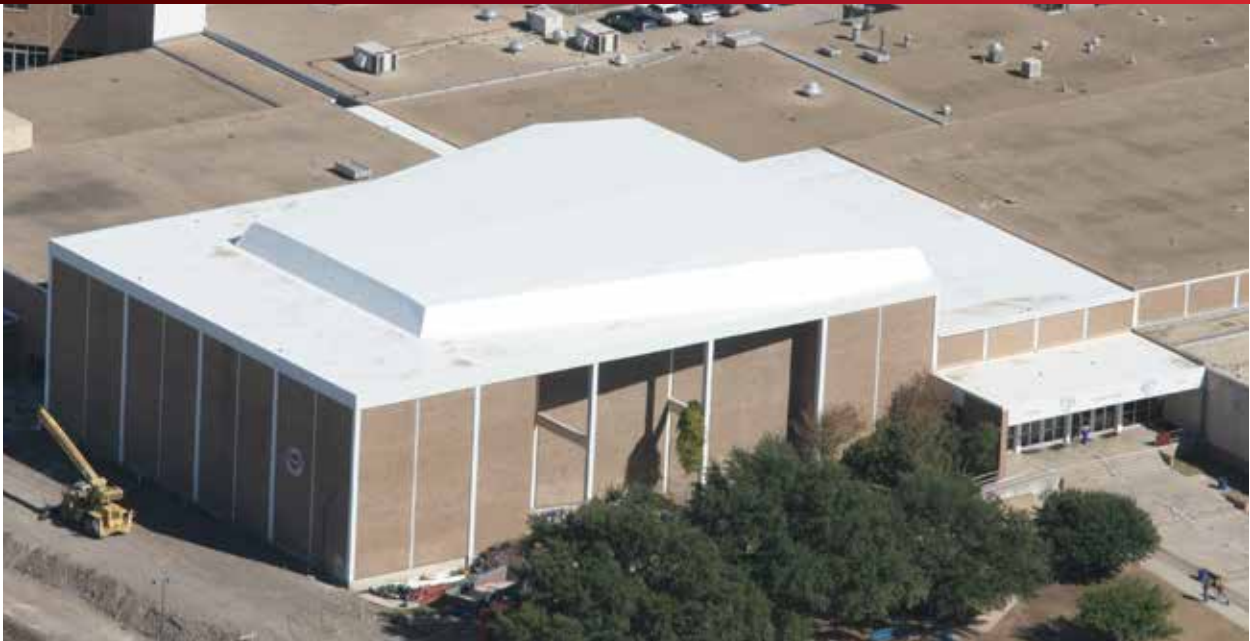
Temple ISD - Scott Elementary - Installed in 2020
