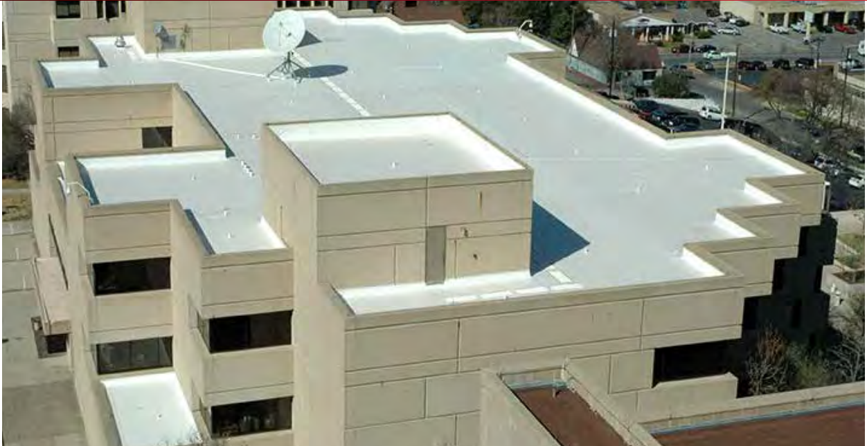
University of Texas - Arlington, TX - Installed in 2011
