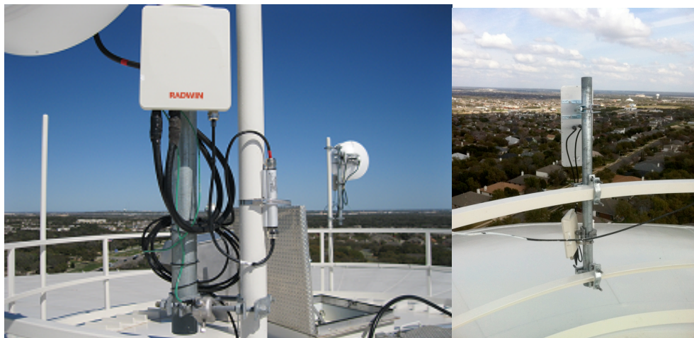
RADWIN wireless systems deployed by regional water utility for SCADA communications
