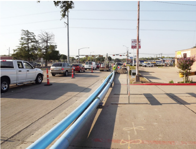
Great value in a contractor being able to upsize a water main while still allowing traffic to flow
