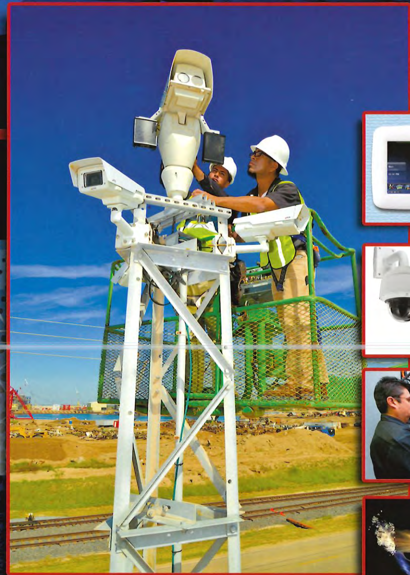
American Surveillance crews servicing video surveillance cameras on a 30-ft Systems tower at the Port of Brownsville.
