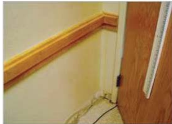
After the room was treated with the hydrogen peroxide gas process, the same wall shows the mold and mildew have been eliminated.
